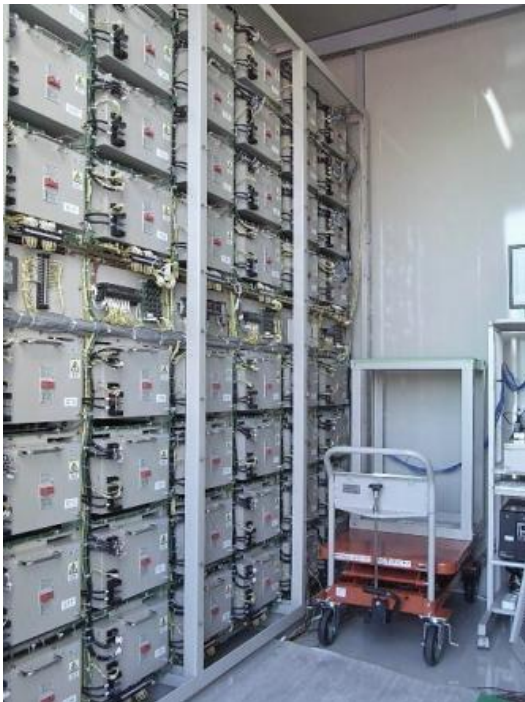
<Interior of the system: lithium ion capacitor board>
