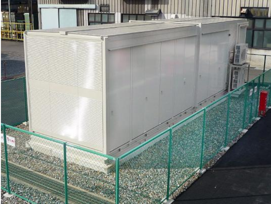
<Exterior of lithium-ion capacitor-based system for compensation of short-term power disruptions:>
