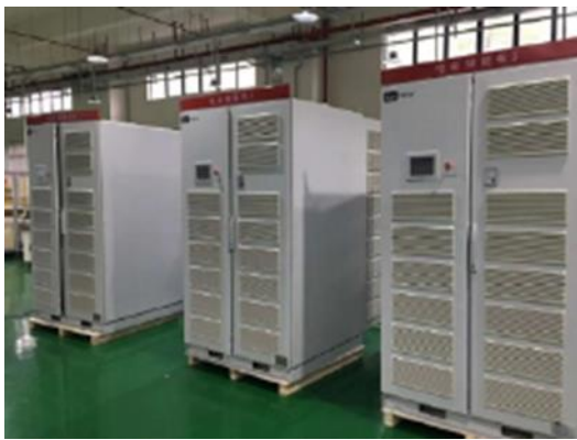
Xīnfēngguāng Wayside ESS
